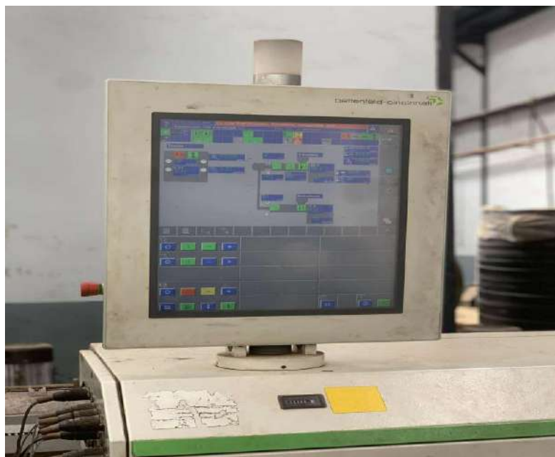
Figure III.15 : Ecran tactile de supervision.
