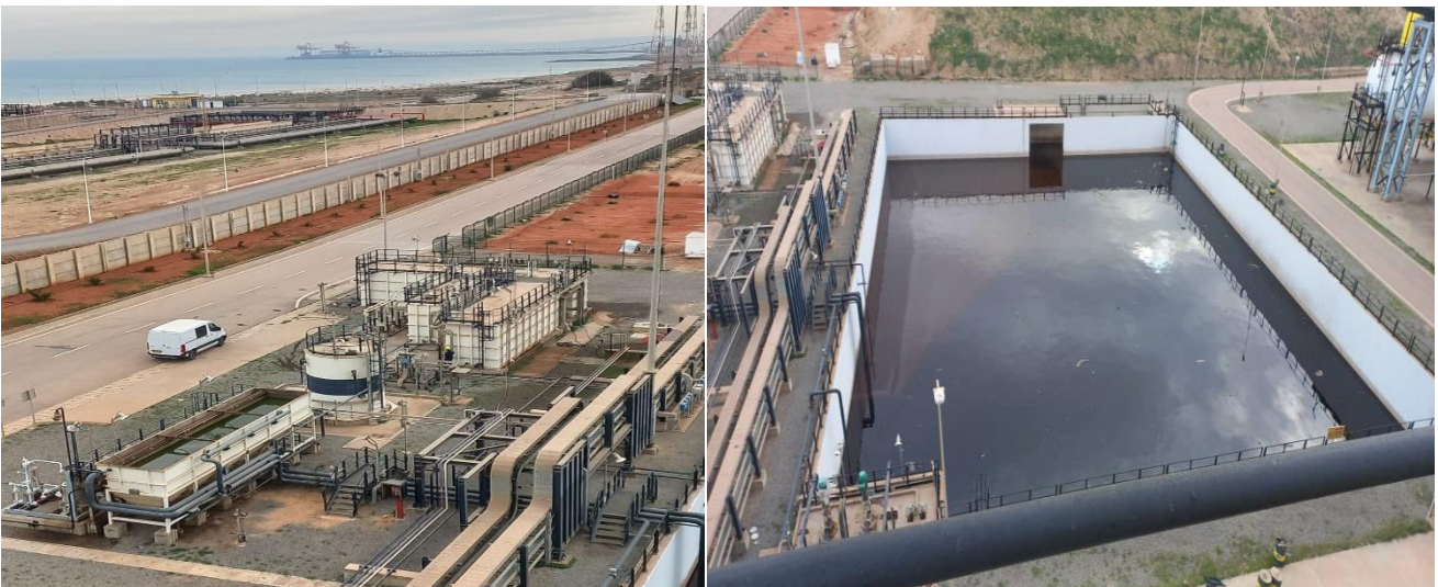
Figure II.2. Water treatment plant (unit 64).
