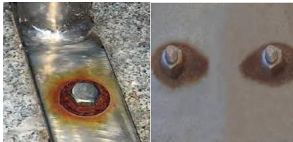
Figure I.7: La corrosion galvanique
