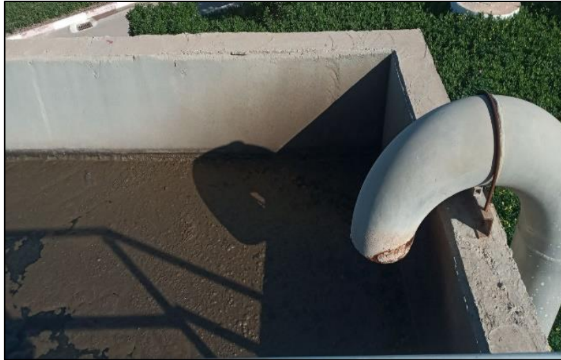
Figure II- 7: Bassin de contact
