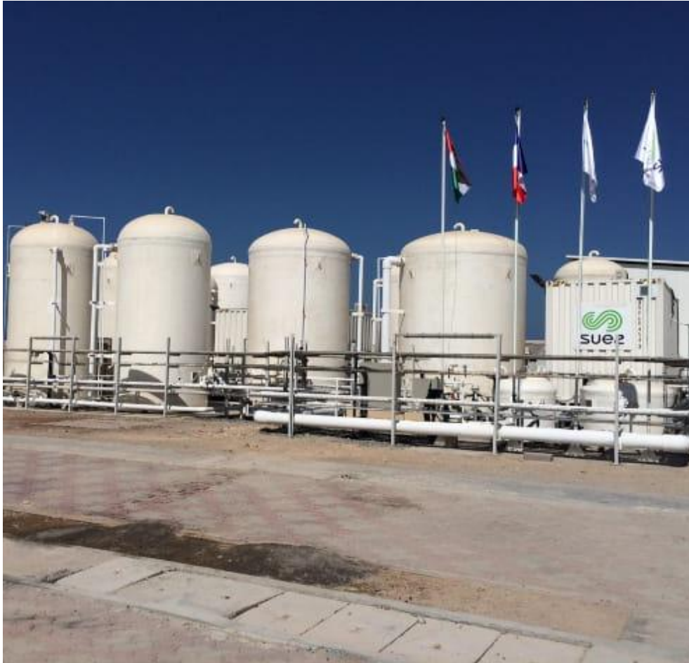
Figure 14 :Ghantoot Desalination Plant (masdar, 2025)
