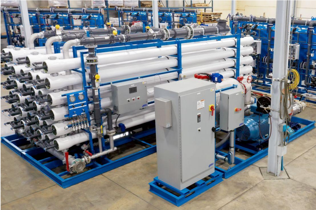
Figure 7 : REVERSE OSMOSIS MEMBRANES
