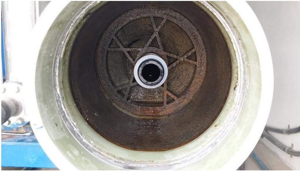
Figure 16 : Damaged membrane due to high salinity (BWC, 2025)
