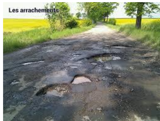
Figure 24: arrachements de chaussée [5].
