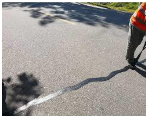
Figure 28: Fissures de joint [5].
