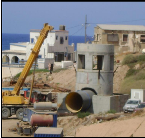
Figure 17: Tour de captage
