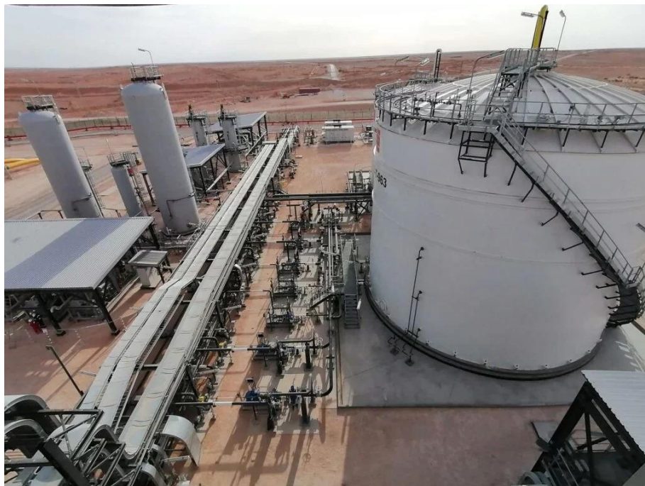
Figure I.4. Module Processing Plant 3 Hassi-R'mel [w3].
