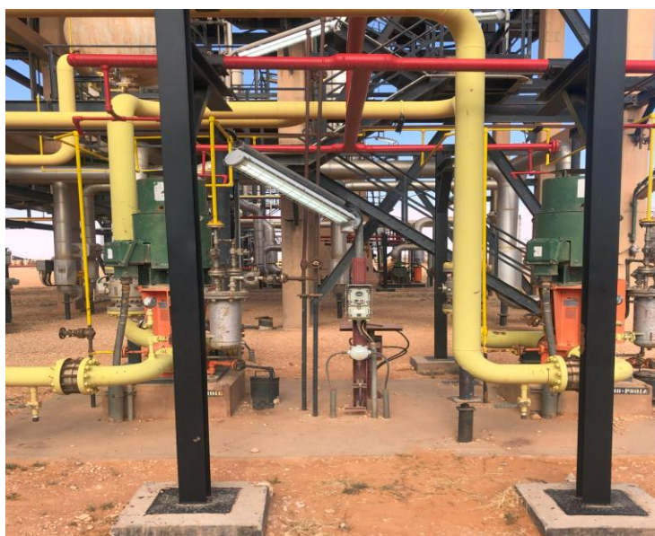
Figure II.5. Centrifugal Pumps Installed in the Depropanizer Unit.
