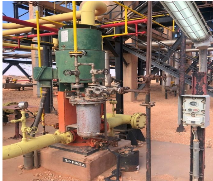
Figure II.4. Centrifugal Pump 38-P-801A Installed in the Depropanizer Unit.
