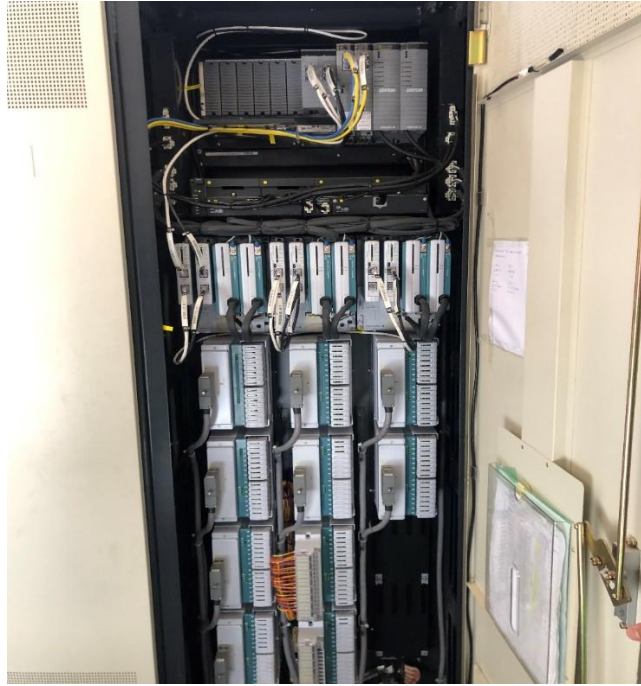
Figure III.4. The FCS station
