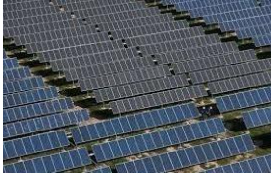
Figure 1.6 Photovoltaic solar power plant
