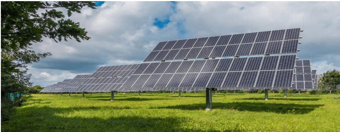
Figure (I.2): Panneaux photovoltaïques
