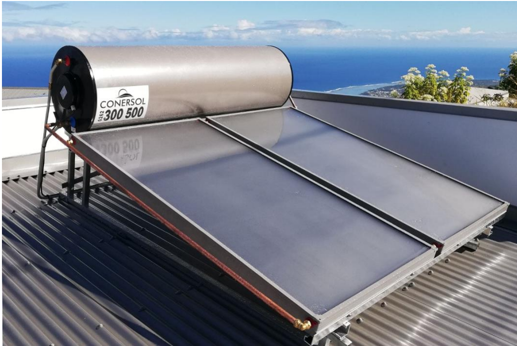
Figure I. 9: le chauffe-eau solaire
