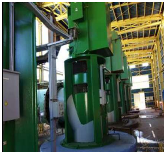
Figure (II.13) : Station pompage E40.
