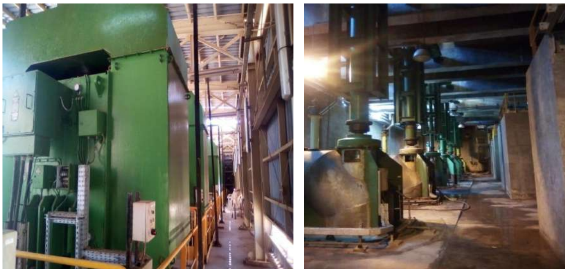
Figure (III.4) : La station de pompage.
