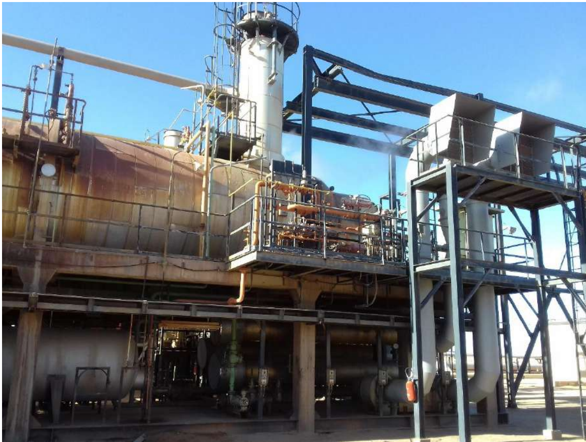
Figure II.1.b. Real picture of Boiler H301
