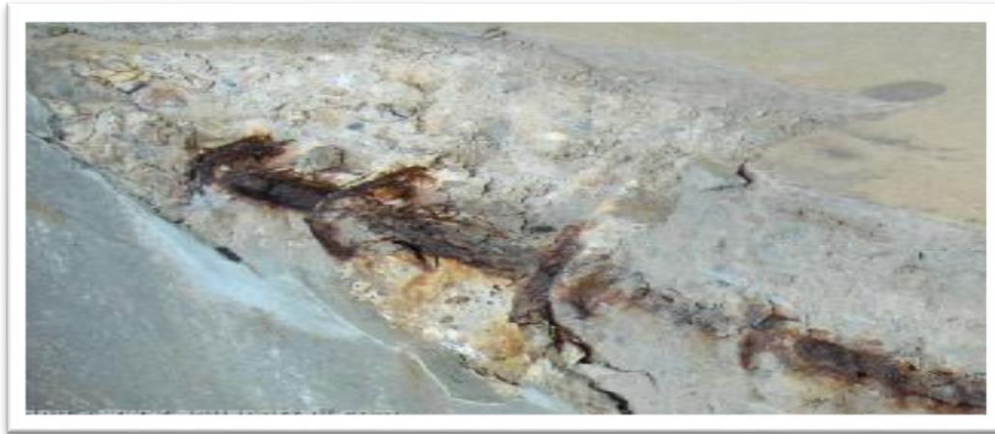
Figure 1. 2 Carbonatation de béton [8]
