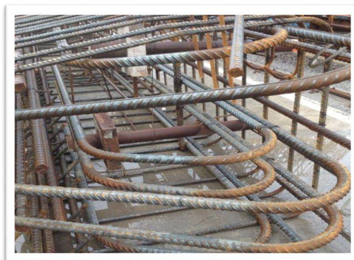
Figure 1. 10 La corrosion des armatures [7]
