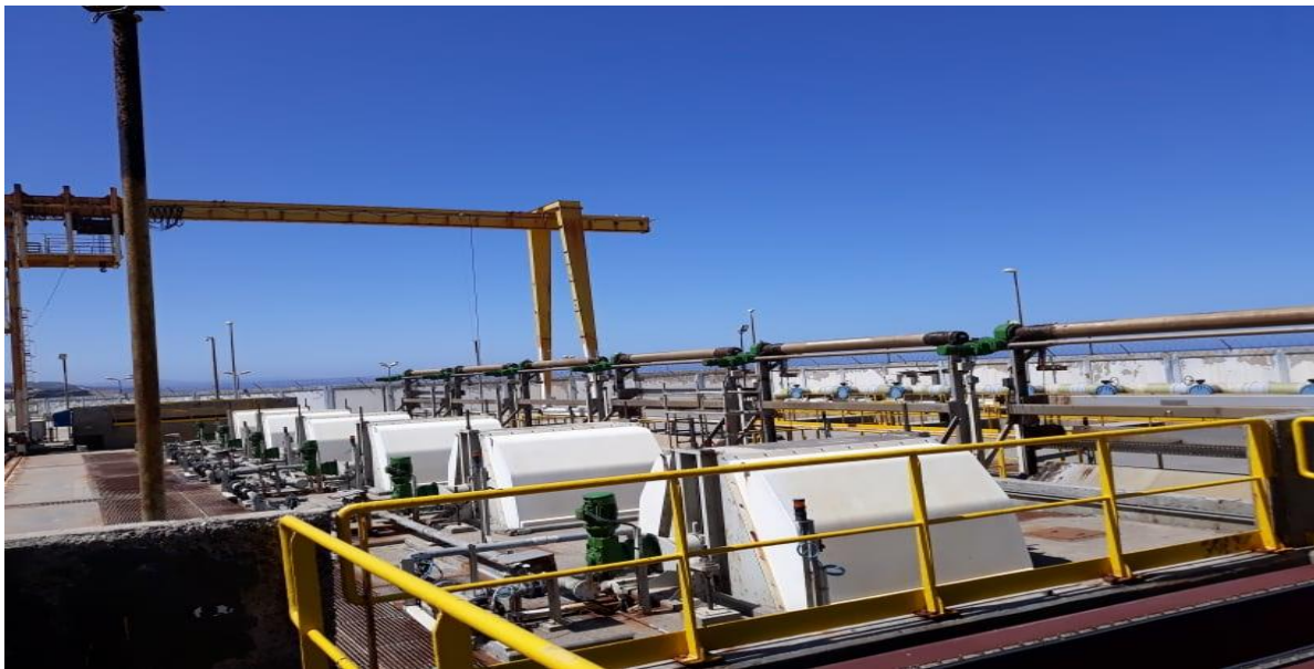
Figure 11 stations de pompages
