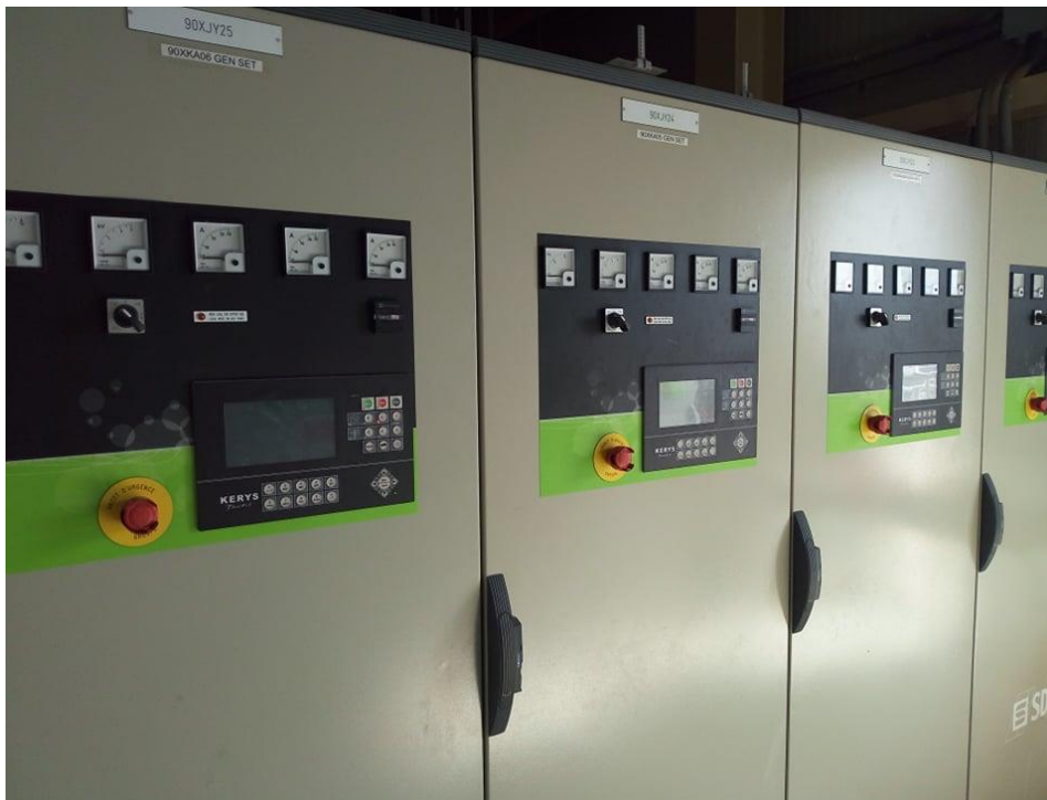
Figure 19 tableaux de distribution BT
