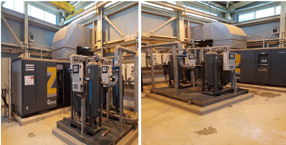
Figure 16 Station d'air comprimé
