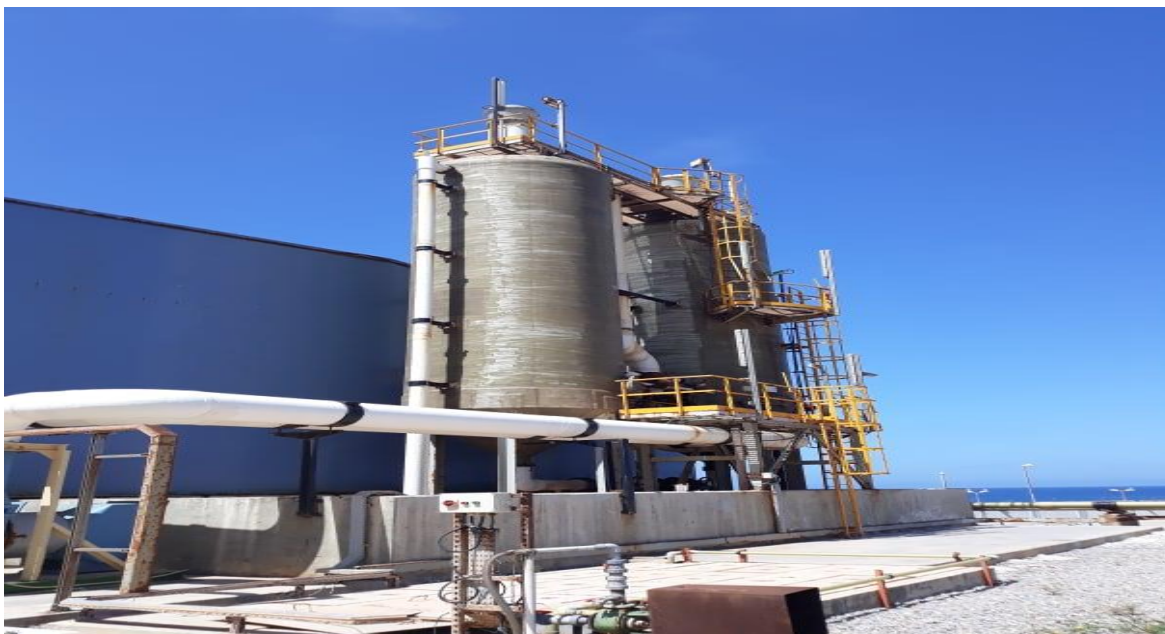
Figure 22 Bacs de stockage
