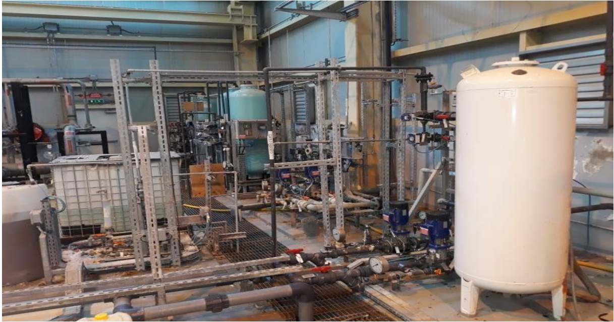
Figure 14 stations de production eau potable
