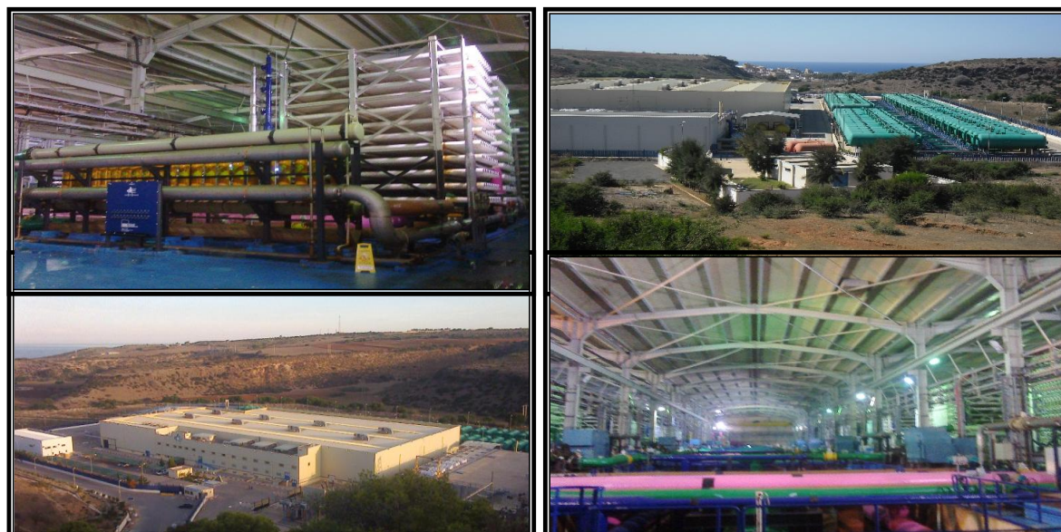
Figure II.8 : Station de dessalement de CHATT EL HILLAL [2]
