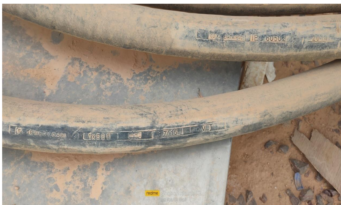
Figure VII.70 : Câble section 500mm 2
