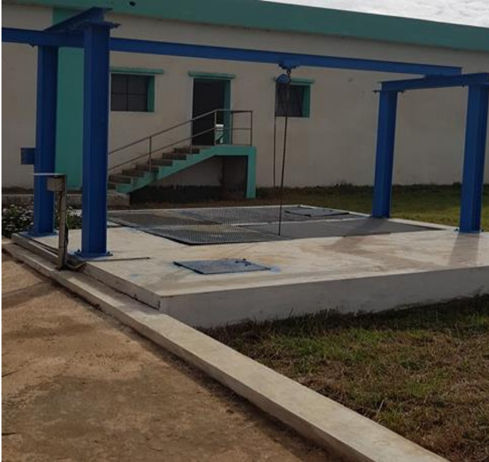
Figure III.23: Puits de drainage.
