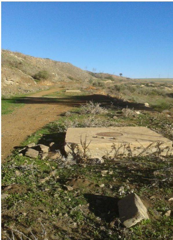
Figure II.6 : Regard de visite
