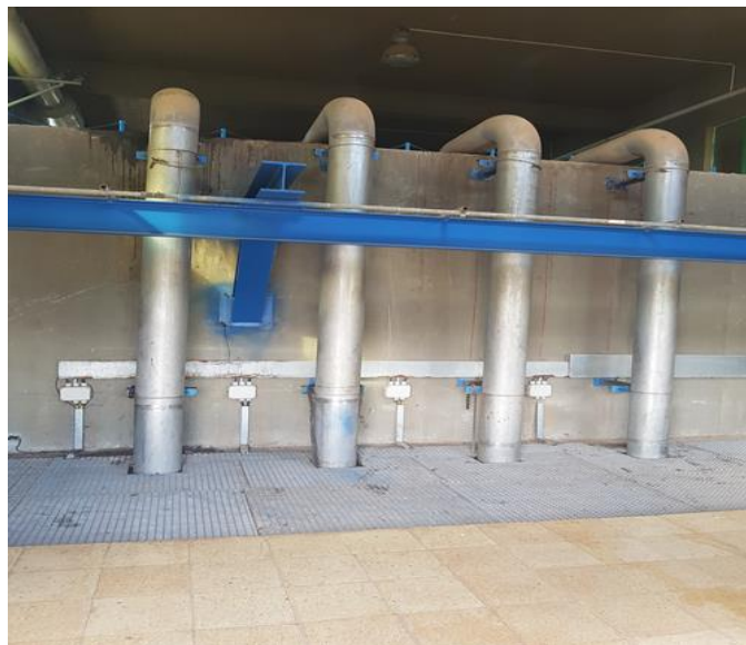
Figure III.10: Station de relevage.
