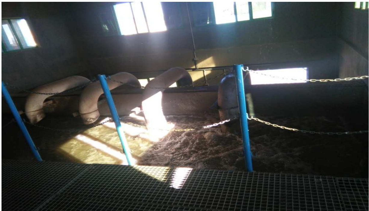
Figure N° 5: Station de relevage
