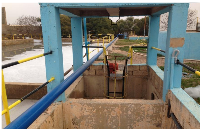
Figure 10 : Station de relevage
