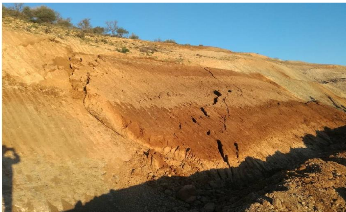
Figure III. 10 Pied du talus PK8+195 a PK8+250 [28]
