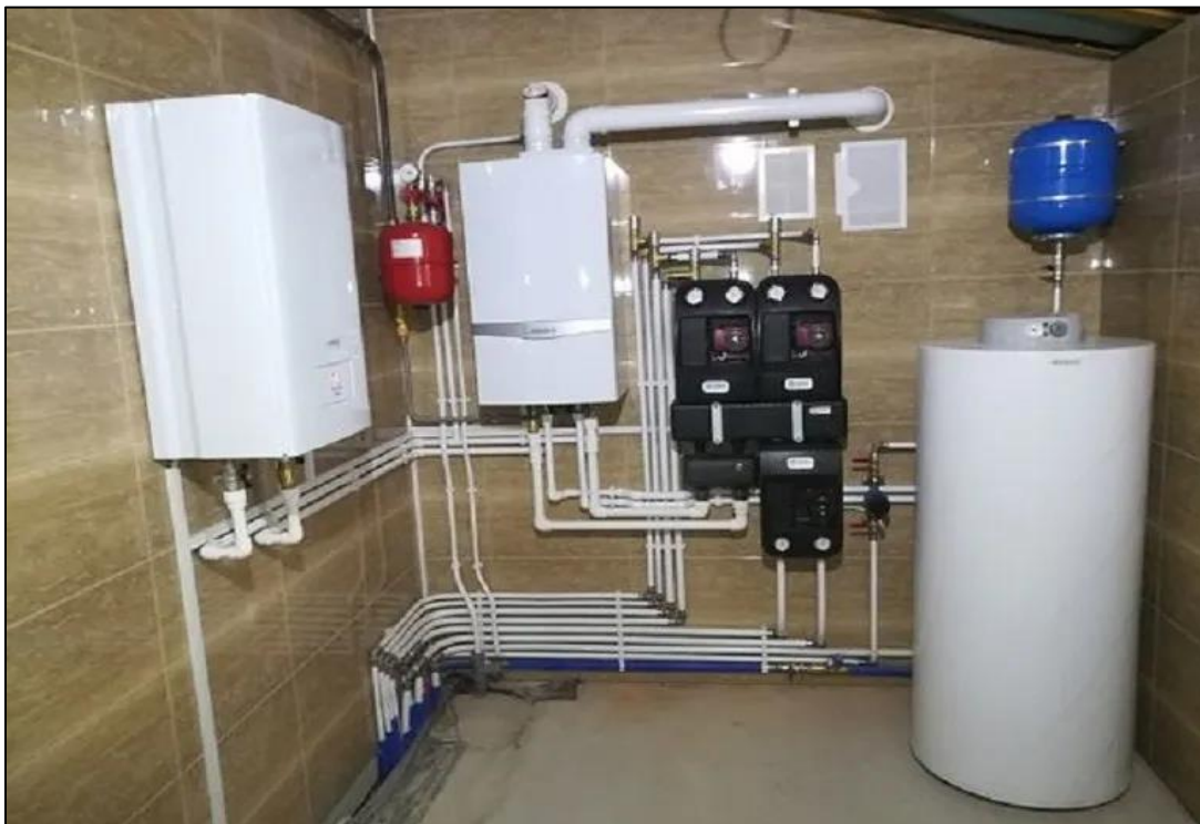
Figure 43: Installation de chauffage central
