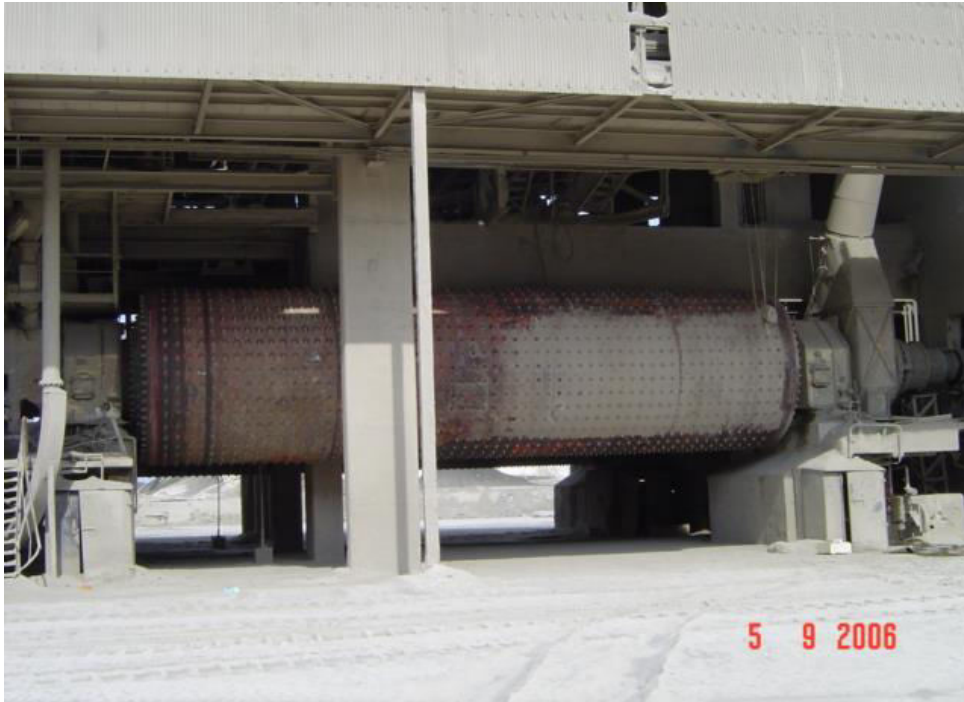
Figure : I.B.9 Broyeur ciment [21]
