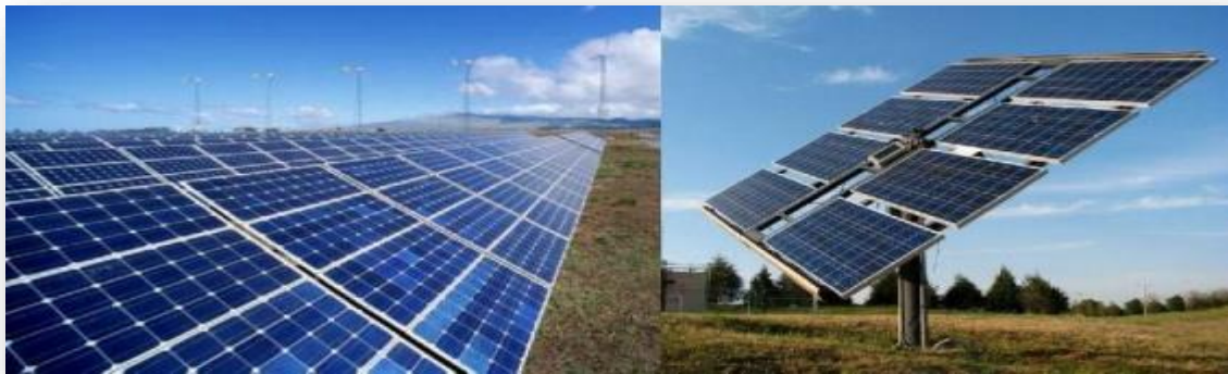
Figure (I.19) : Panneau photovoltaïque .
