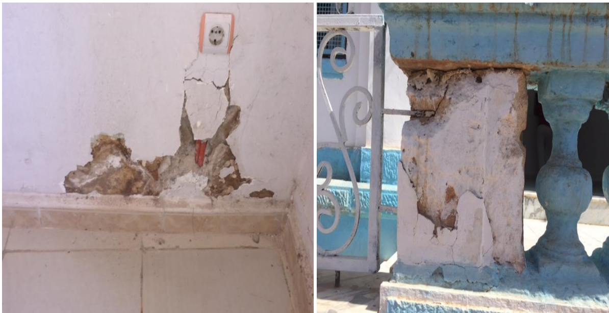
Figure III.22 : La desquamation de la pierre
