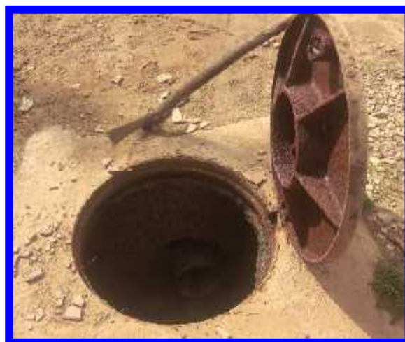
FIGURE 10 : REGARD EXISTANT DEGRADE
