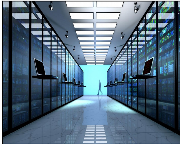
Figure (I.2) : Data center [8].
