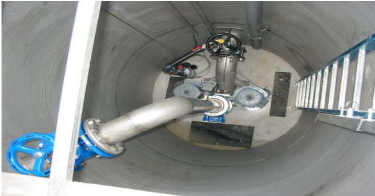
Figure 13: Station de relevage
